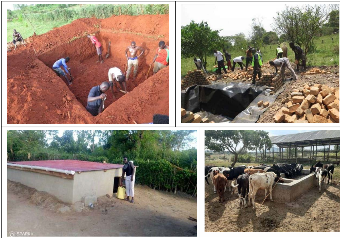
Figure 10. Field photos for construction of water facilities at Mrs. Tumuhairwe Robinah's farm, a beneficiary beef farmer in Kyankwanzi district, Uganda
